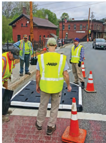
◀ MAIN STREET, BETHEL, VERMONT: During the Bethel Better Block pop-up demonstration event in 2016 (far left), bulbout curb extensions were crafted out of straw-filled wattles encircling potted plants. Soon after, rubber bulbouts (left) were installed along the roadway.
