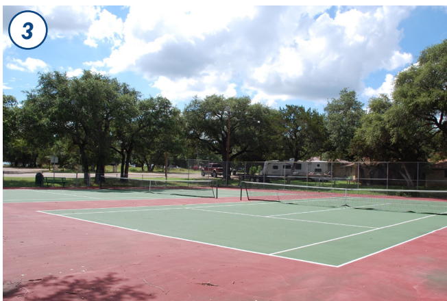
The existing tennis courts are in need of maintenance.
