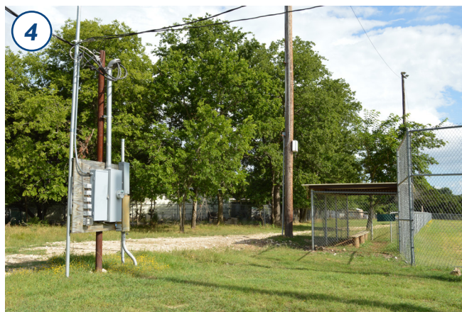
The electric utility boxes create a potential safety hazard.
